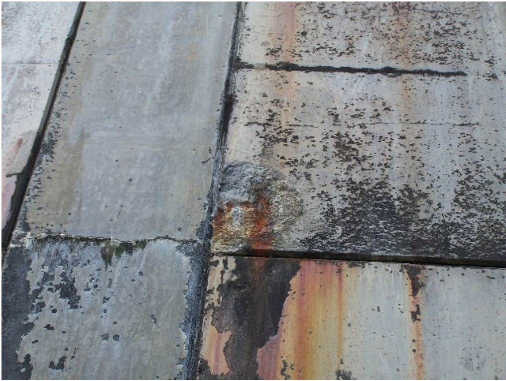
Plate T6: Close-up of a typical rust stain, with associated surface spalling at the corner of a panel.
