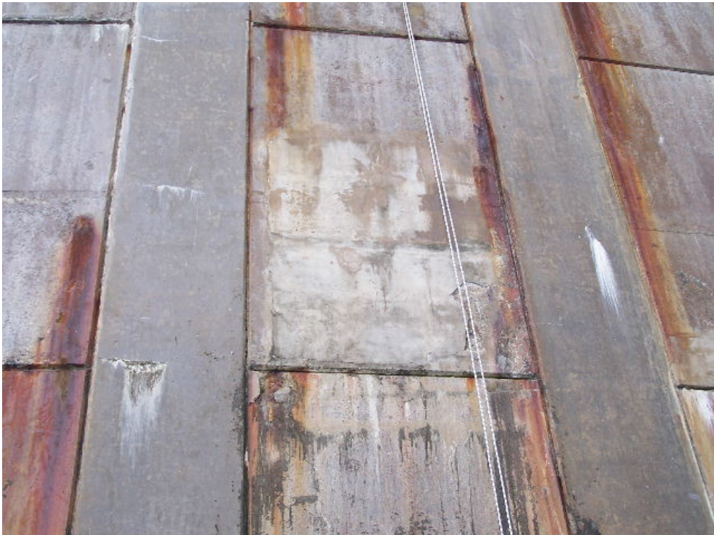
Plate T7: Close-up of previous patch-repair. Many were found to be hollow and delaminated.
