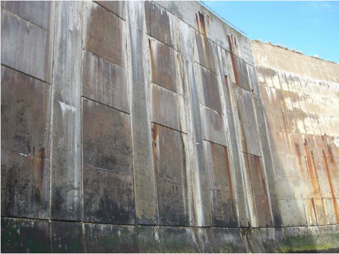
Plate T3: Close-up of the wall showing pre-cast columns, separated by discrete panels. Rust staining was widespread.
