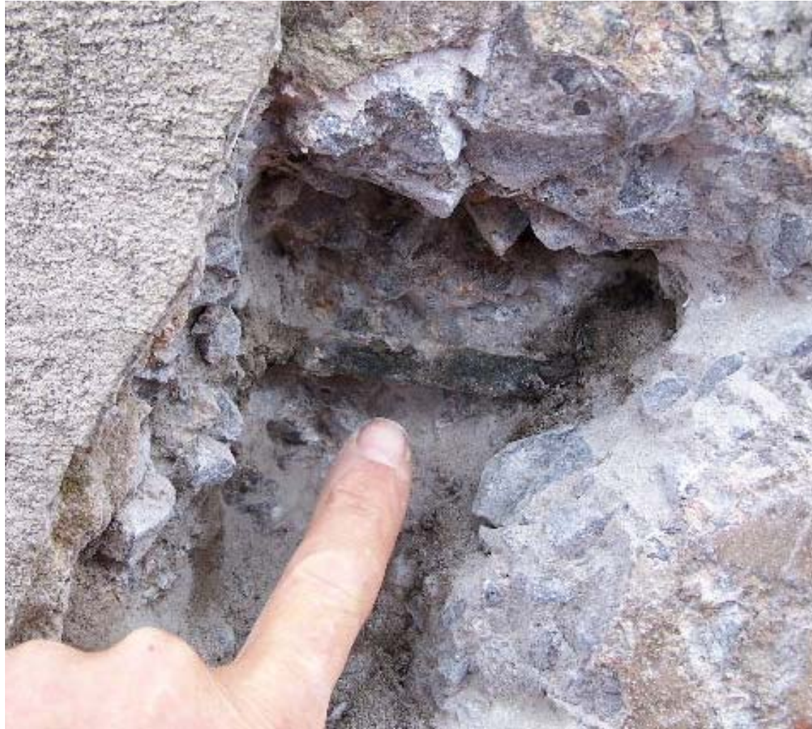
Very Badly Corroded 10mm Horizontal Bar
