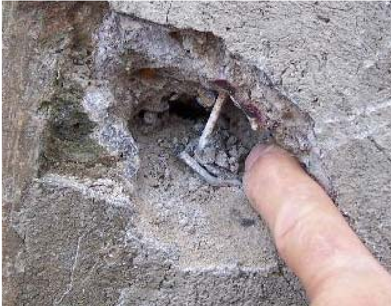
Surface Corrosion on the 2mm Mesh in the Previous Repair Patch
