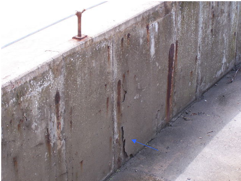
Plate T8: General rust staining and spalling (arrowed) on the inside of the parapet wall.
