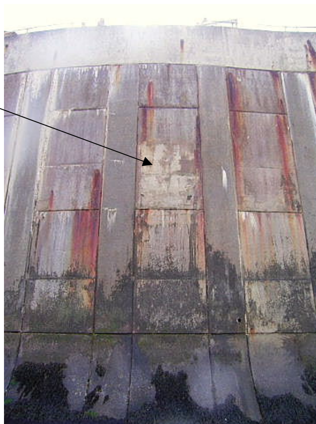
Plate T5: General view of Panels 29, 30 and 31 showing various types of 'defect' i.e. cracking, previous patch-repair, rust stains and white deposits.
