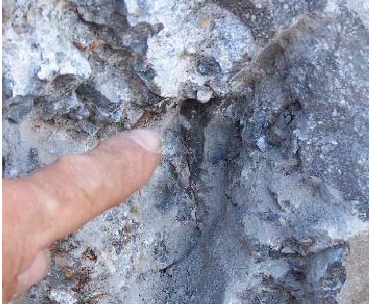
Very Badly Corroded Vertical Bar.
