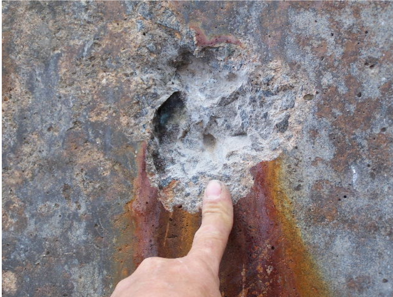
Break-out at Rust Stain to Reveal Degraded Pyritous Aggregates Particle .
